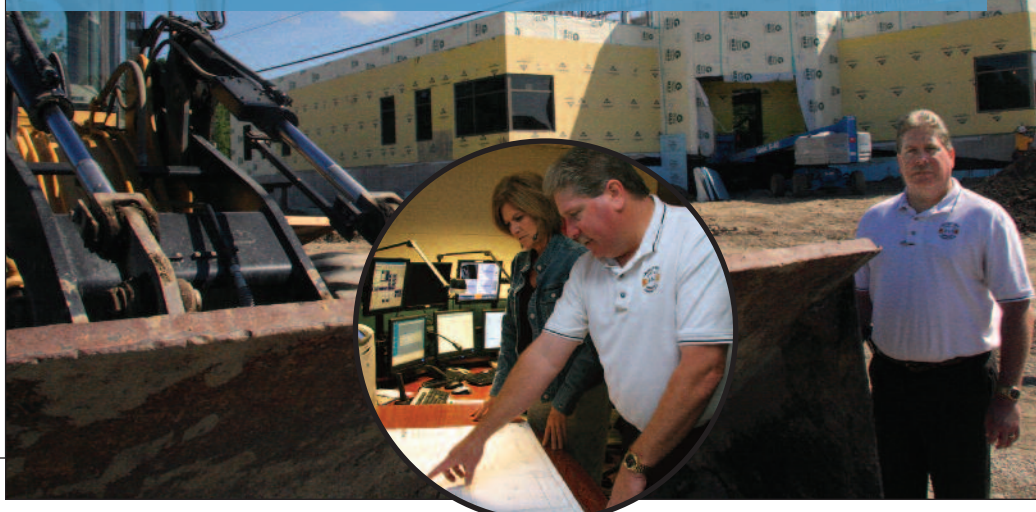
Brad Veerman, deputy director of the Lincolnway Public Safety Communications Center, visits the construction site for Frankfort Township's new administrative building, where the Lincolnway PSAP and its radio room will be relocating in December. Inset: Veerman shows Telecommunicator Teri Killian the blueprints for the PSAP's new radio room.
